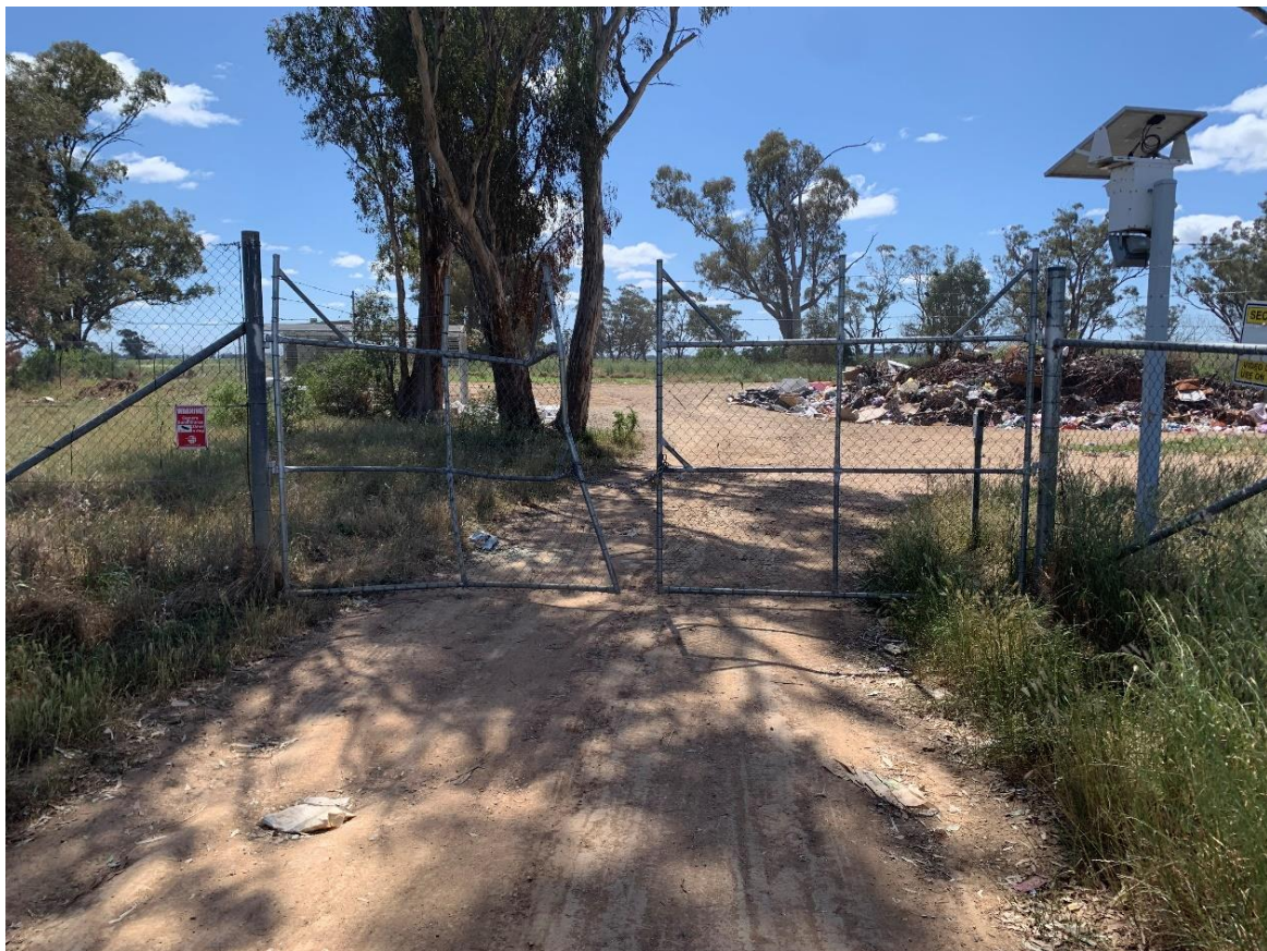
Figure 2. Damaged cause to front gate at Quandialla facility.
