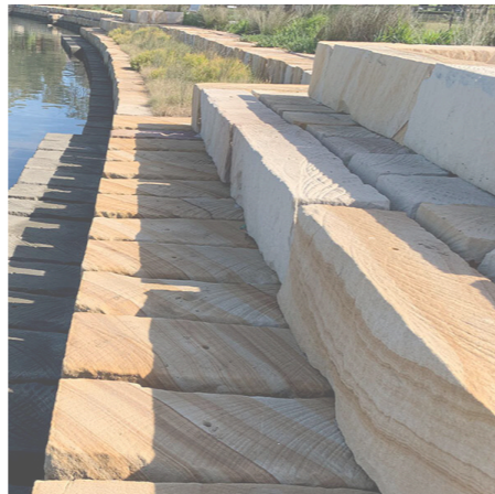
4 Stacking of sandstone blocks for youth perching and seating from a vantage point.
